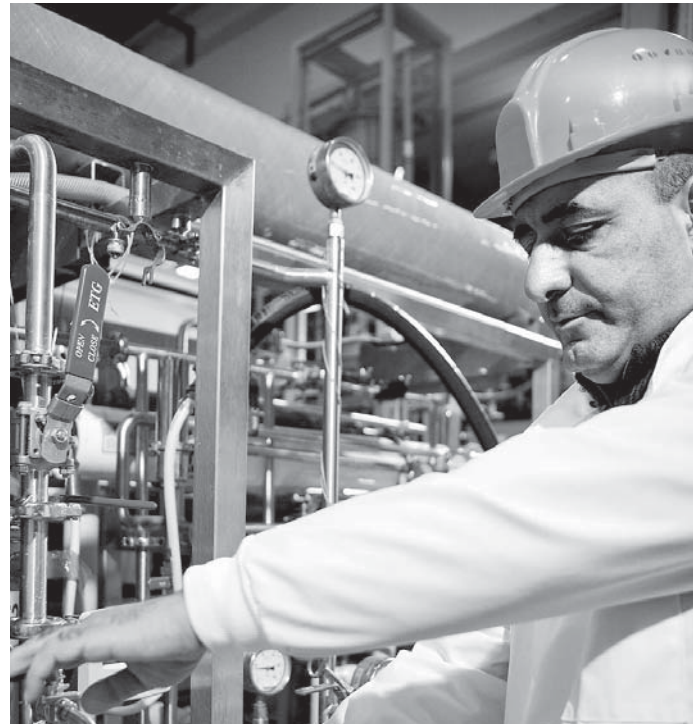
Modern Water uses a desalination process called 'manipulated osmosis technology'
