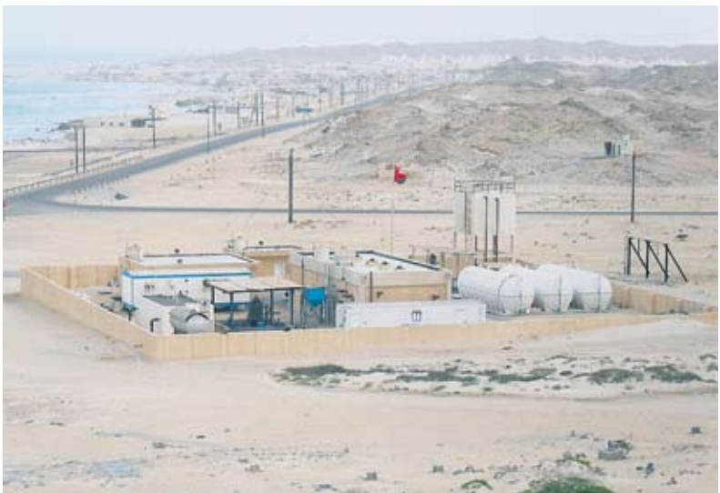
Modern Water has set up a desalination plant in the Al Khaluf region of Oman
